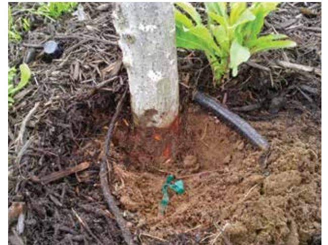
Do not bury the top main root, expose the root flare above grade.
