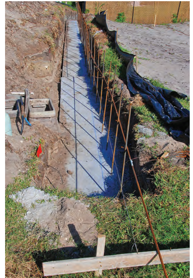
Above: This footer for a retaining wall will block tree roots and stunt growth.
