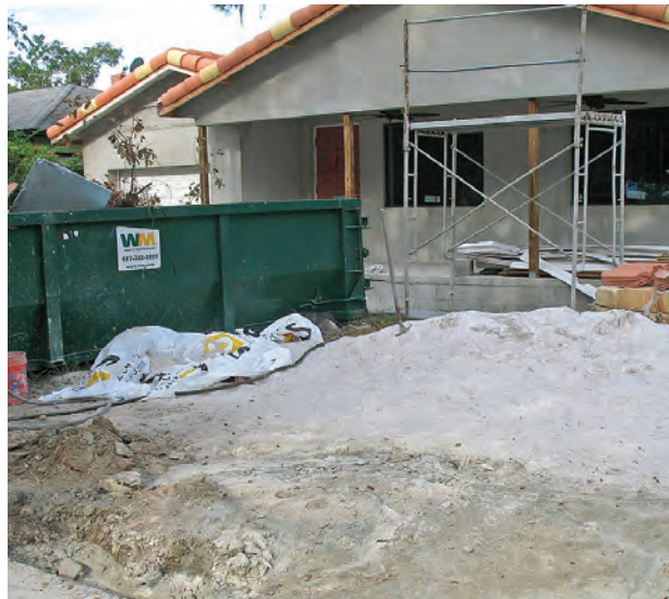
Above: These soils are contaminated with construction materials.
